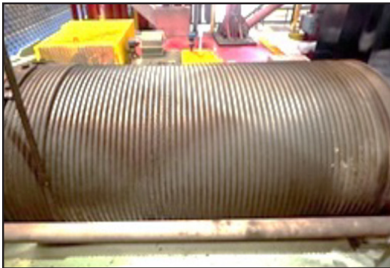
Wire rope hoist system inside the steel mill for moving stainless steel coils inside the plant.
